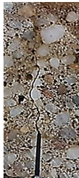
Figure 3 (a) An example of a load-displacement curve, (b) SENB testing setup for conducting fracture test on PC mixture, and (c) the failure path and crack growth
